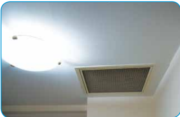
Air-conditioning systems are among the means by which smoke can drift throughout a building
